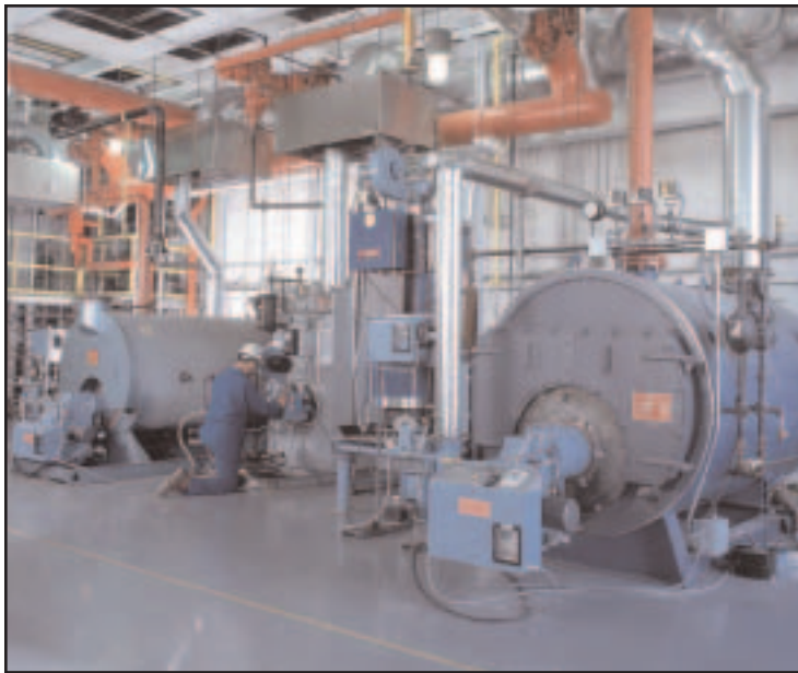
A boiler room test bay at John Zink Co.’s Research and Development Test Center where Gordon-Piatt boilers are tested.
