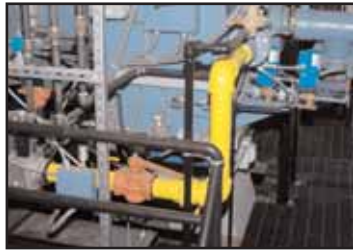
The Wilkinson Centurian, pictured here at NU, is comprised of a Gordon-Piatt burner, the Autoflame combustion management system and a Hurst boiler.
