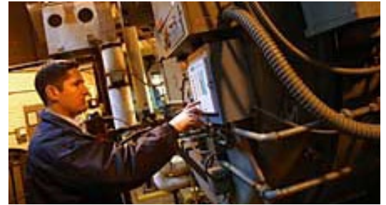
Geoffrey Wilkinson Jr. looks over an Autoflame control panel retrofitted to an older boiler at Northeastern University. (GREG DERR/The Patriot Ledger)
